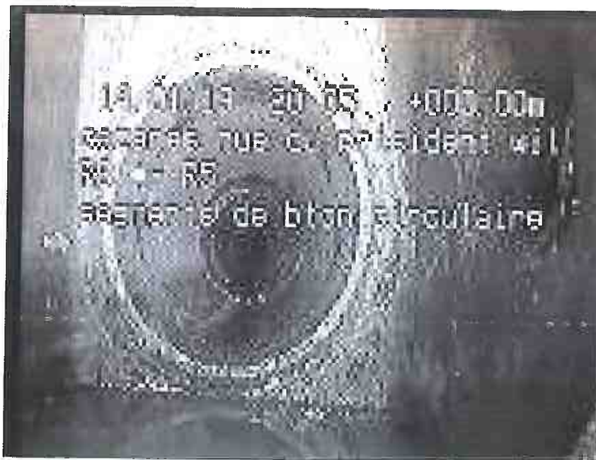
Photo: 10_10_44_A.JPG, N° support: 2-14012018 c_7 0m,
